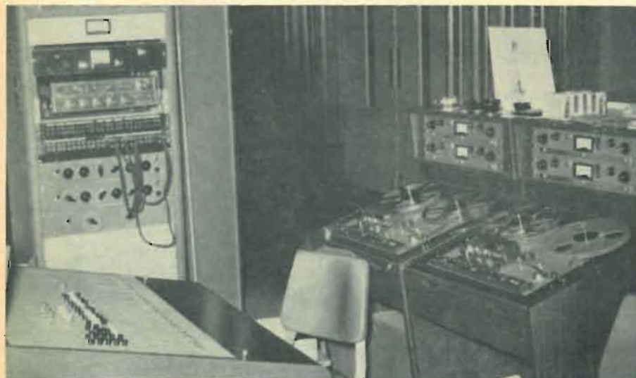
The system set up and ready for use, with console at left. Rack contains limiter, feedback stabilizer, equalizers and power amplifiers. Tape machines record the proceedings.
